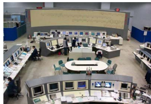
Figure 14. The Control Center Room in Taipei MRT
