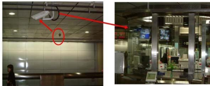
Figure 19. The CCTV and fire alarm systems in underground stations' public area interlocked
