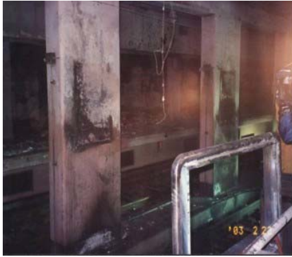
Figure 1. The underground third floor of track zone in the subway Jungangon Station
