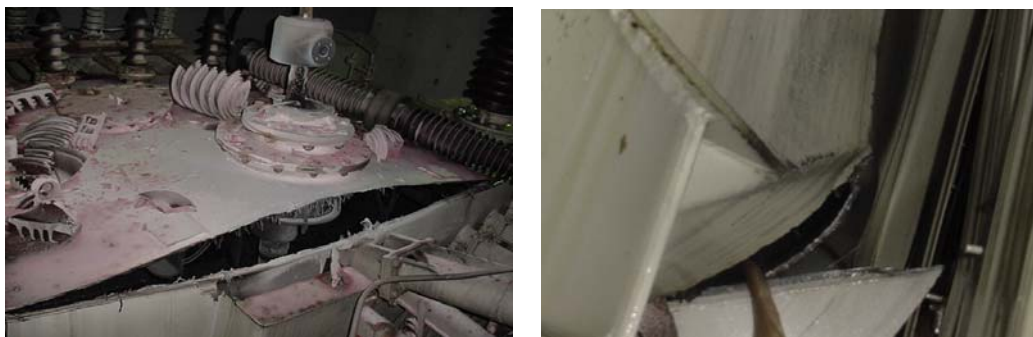
Fig.1 Damaged part of transformers
