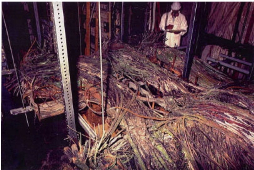
Figure 7. Burned cables in Hinsdale telephone exchange fire, reproduced with permission from FTI report [12].
