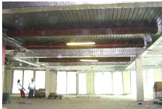
Fig. 5. Unprotected secondary steel beams at Plantation Place South, London as a result of FE analysis of the frame in fire.
