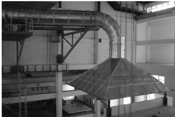
Fig. 1. Fire products suction cone and pipeline.
