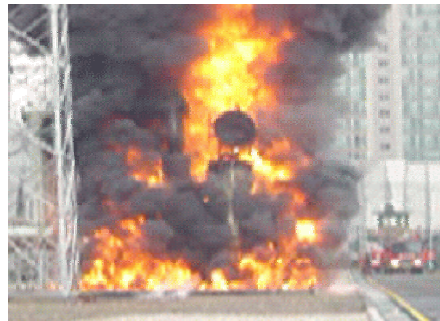
Fig. 2. Transformer fire incident.
