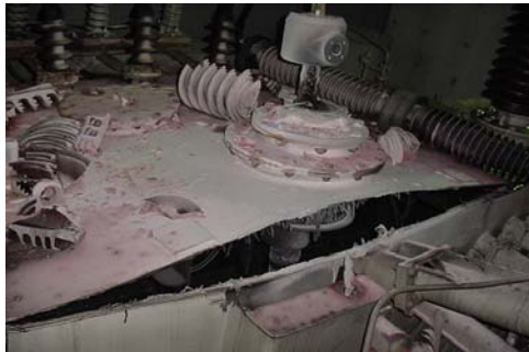
Fig. 1. Damaged portion of the transformer.
