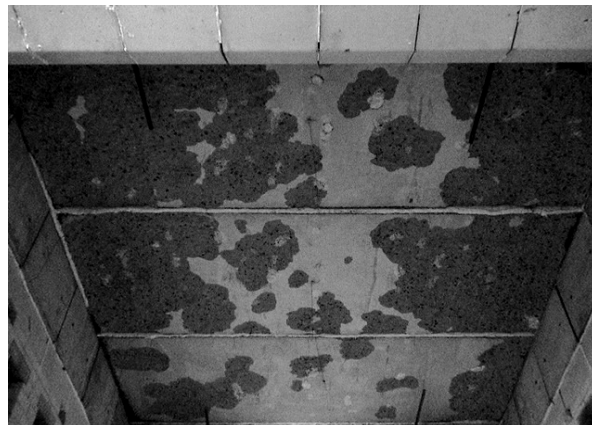
Fig. 3. Explosive spalling of slabs S1-S3 (bottom heated surface)
